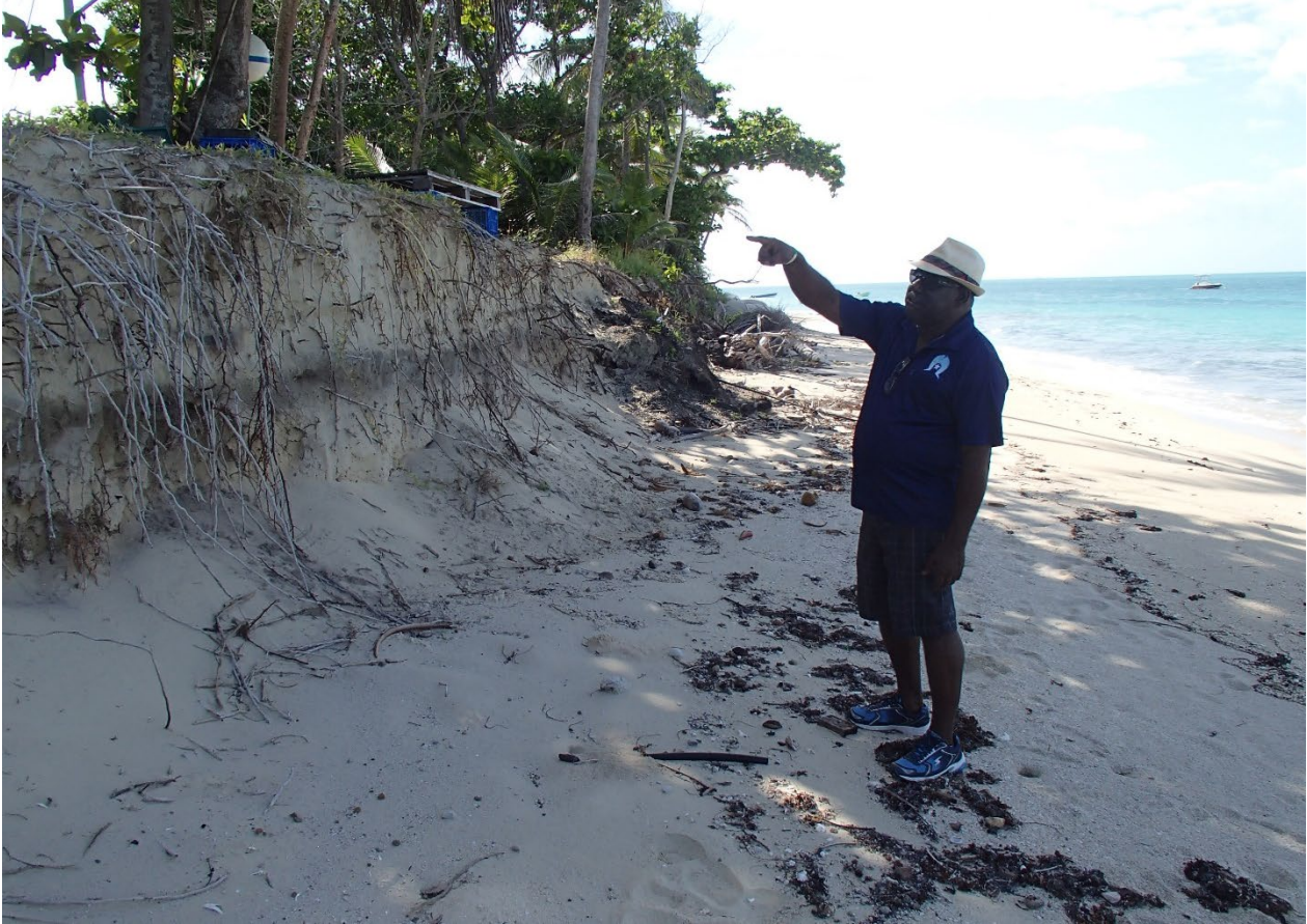
Figure 27 Erosion undermining mature trees on south-west coast of Poruma (February 2018)
